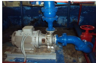
Figure 2 Pump and inlet valve
